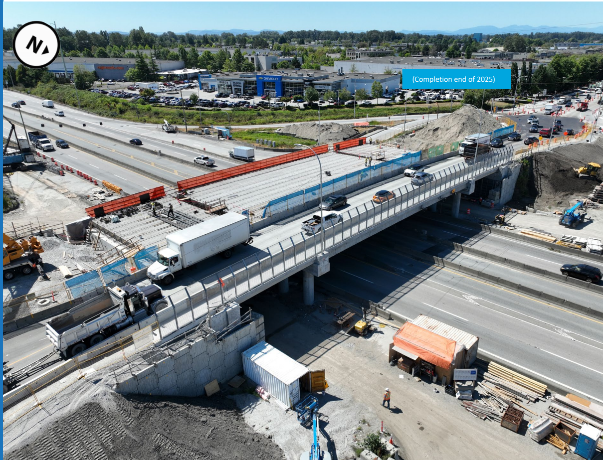
Girder installation on the south portion of the Steveston Interchange Project, August 2025.
